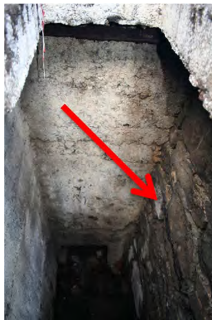
Plate 2.19: 'Tide-mark' on East wall
