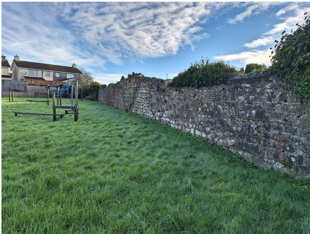
Image 15: Existing south-eastern boundary wall of former Tuam Workhouse onto Tober Jarlath Road
