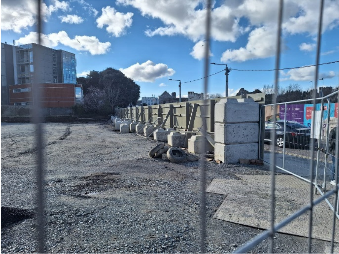
Figure 3: Hoarding supported with concrete Kelly blocks - Avoids the need for excavations for hoarding.
